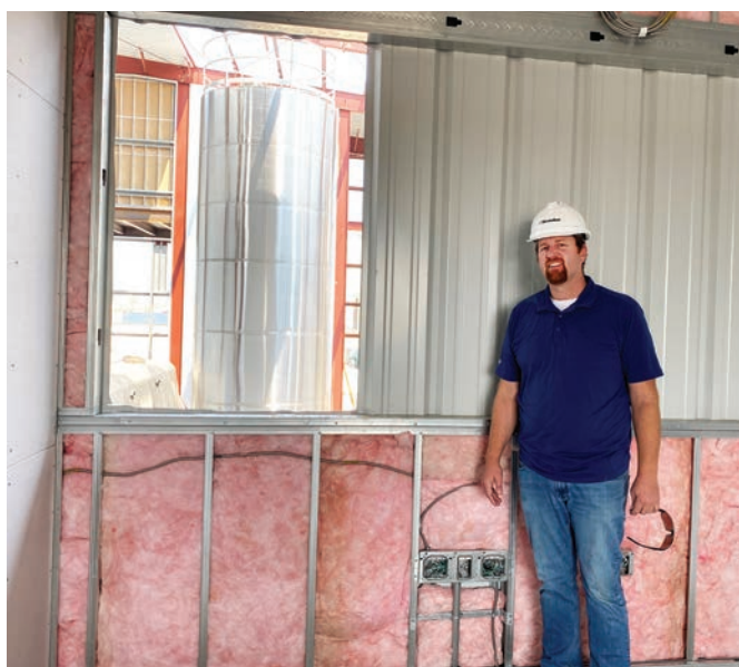
JC Olson checks construction progress at Scoular's new Barley Protein Concentrate Facility on August 3.
