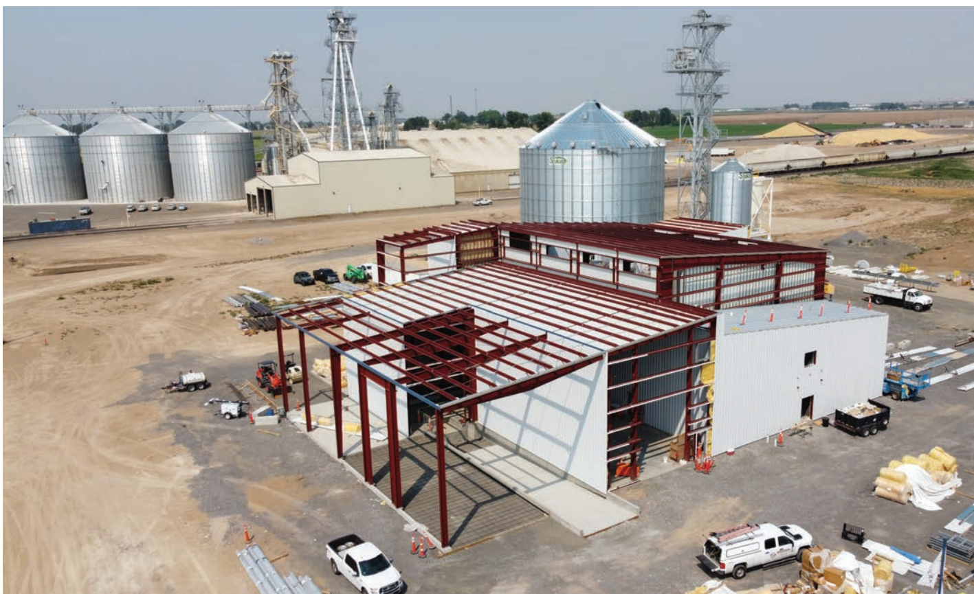
New Scoular Barley Protein Concentrate Facility in Jerome slated to open in mid-October. Photo taken August 3.
